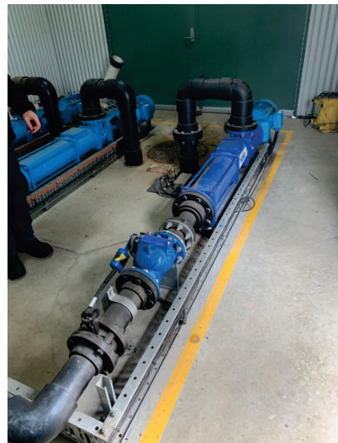
Wastewater network pumps
