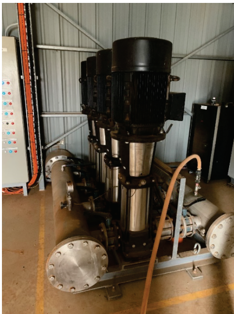
Wastewater treatment plant equipment (treated wastewater pump)
